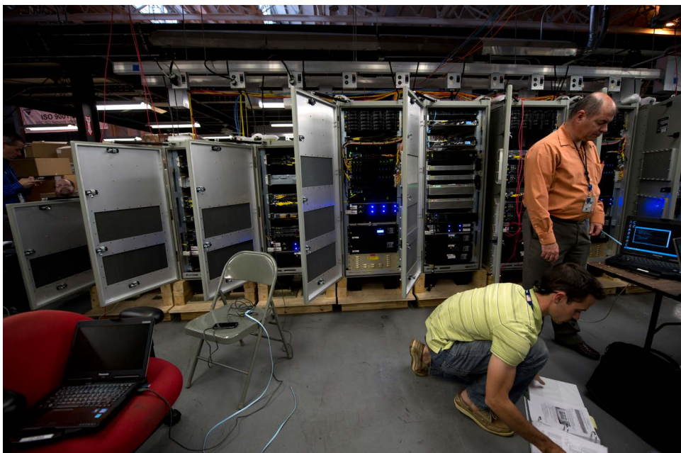
SAN DIEGO (Jan. 23, 2013) CANES technicians at the Space and Naval Warfare Systems Command prepare the system for installation aboard the Arleigh Burke-class guided-missile destroyer USS Milius (DDG 69). (U.S. Navy photo by Mass Communication Specialist 3rd Class Karolina A. Martinez/Released)
